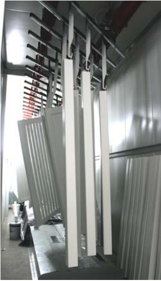
Painted products in drying chamber.
